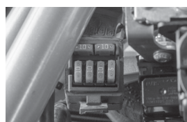
Fuse Box with Cover Open
